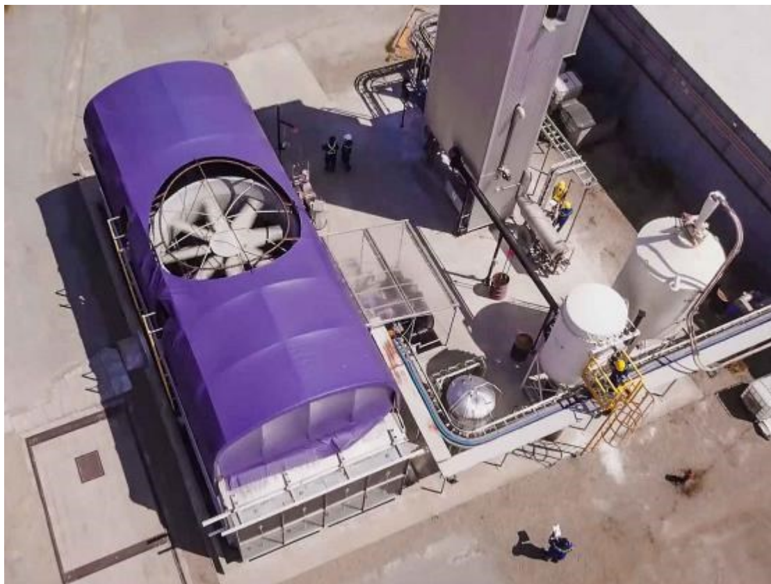
Photo: Carbon Engineering Carbon Engineering is expanding its British Columbia pilot plant to capture 4 metric tons of carbon dioxide per day.
